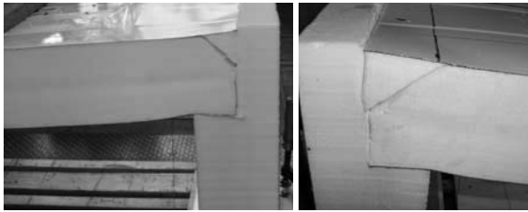
Figure 11: Failure of glued corner details
