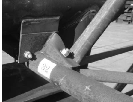
Figure 8: Connection failure of the truss with sleeve connection.
