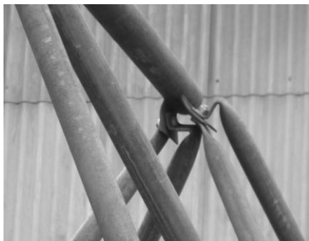
Figure 10: Connection failure of the truss with flange connection.
