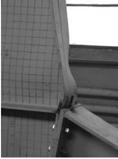
Figure 5a. Failure mode of specimen J2-3m – monotonic loading
