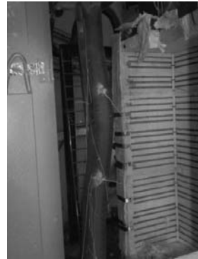
Figure 6: Column E18 after test
